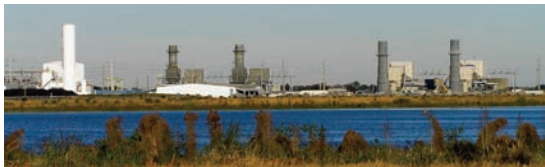
The Polk Power Plant, one of two operating IGCC facilities in the United States
